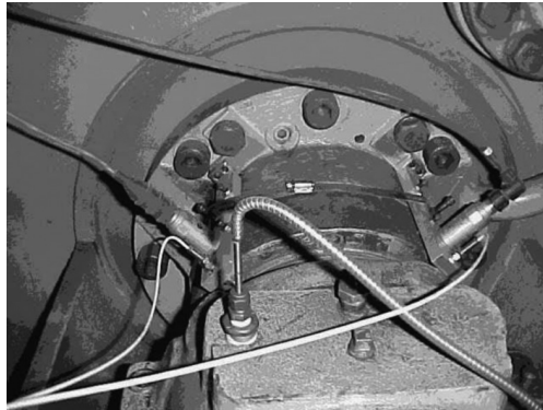
FIGURE 6.6 Retrofitted proximity probes and velocity pickups.
